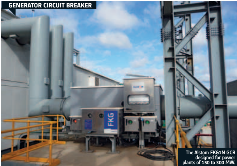
GENERATOR CIRCUIT BREAKER
