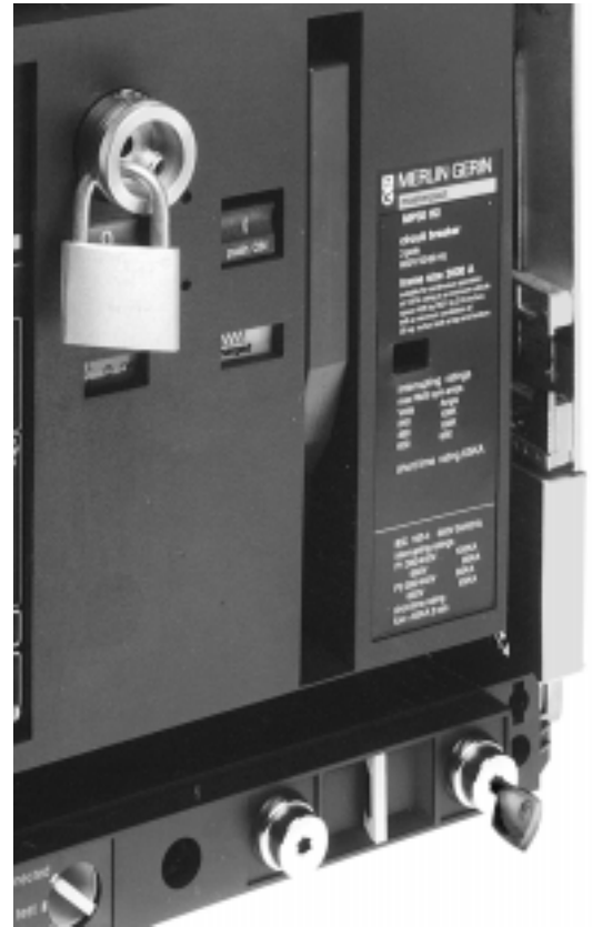
fig. 24: Interlocking devices on a Merlin Gerin Masterpact circuit breaker.
