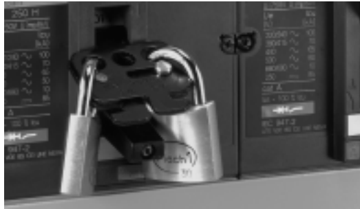
fig. 23: Padlocking device on a Merlin Gerin Compact circuit breaker.
