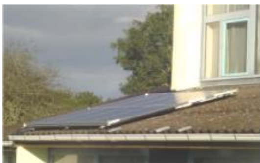
Figure 5 : Panneaux photovoltaïques installés (7 m 2 )
