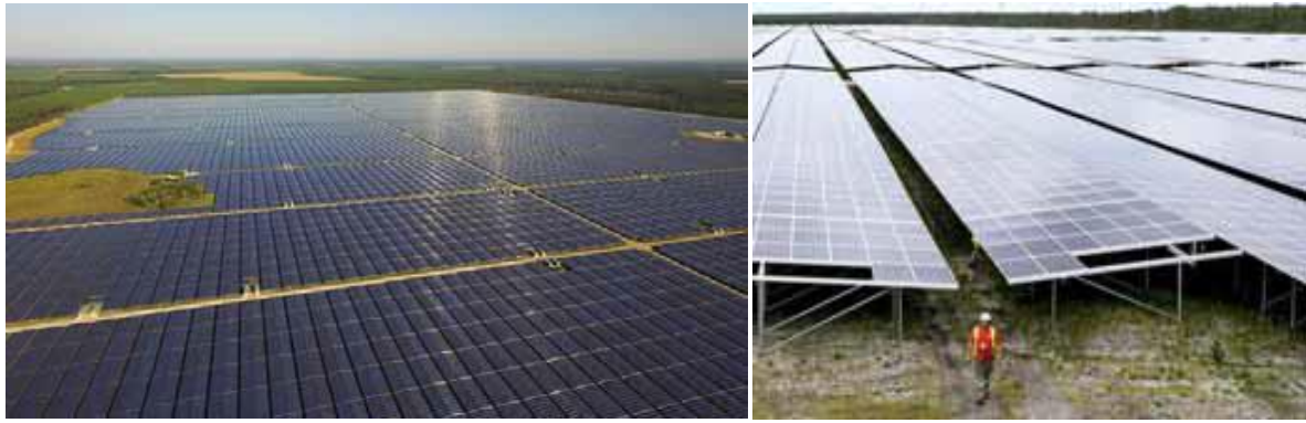
Figure 22 : Centrale photovoltaïque de Cestas (Gironde), source [13]
